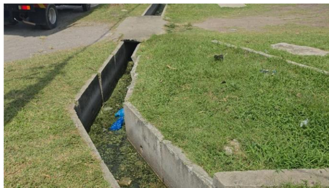
Figure 1. Gutters and the roadside drainage system in the investigation field
