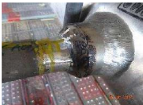
Figure 2. General view of the outlet piping (hairpin) to weldolet (hot collector).
